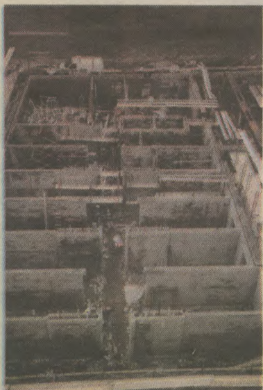
Going up please! A look of the first floor of the new hall. Building started in Sept. '98.
